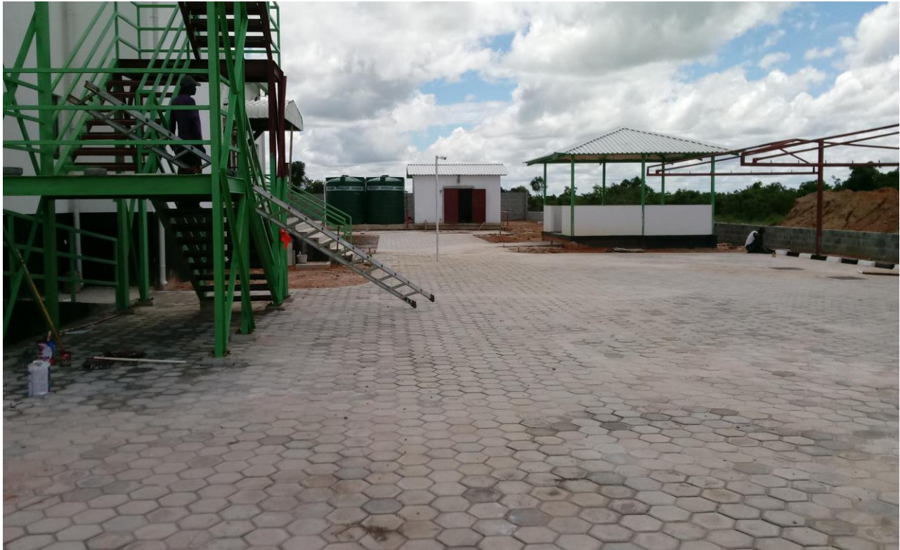
Fig 4 shows the paving, lunch area and pump house at the far end
